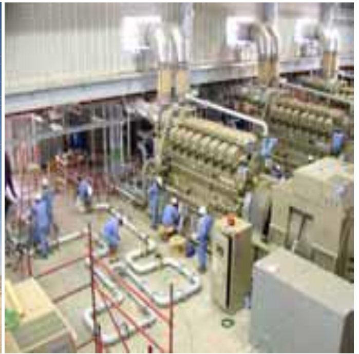
2x 20 MW POWER STATION; MUKALLA CANADIAN NEXEN; YEMEN 2001-2001
