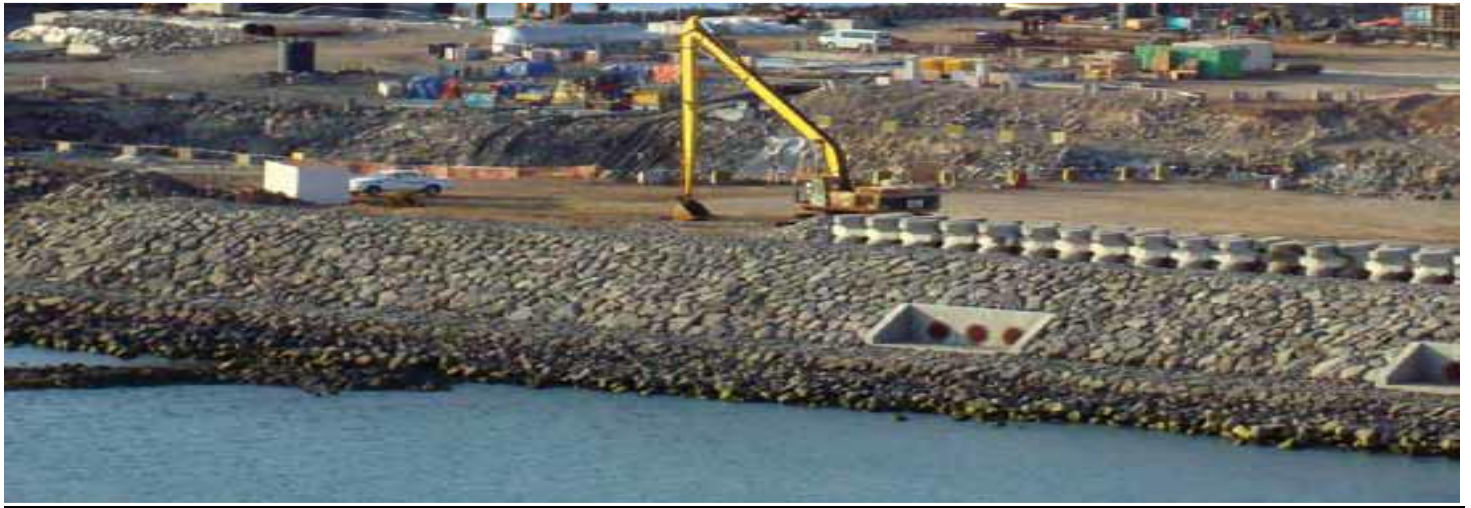
Balhaf Site Preparation & Shore Protection project Project Yemen LNG Plant, Balhaf / Yemen 2006-2010
